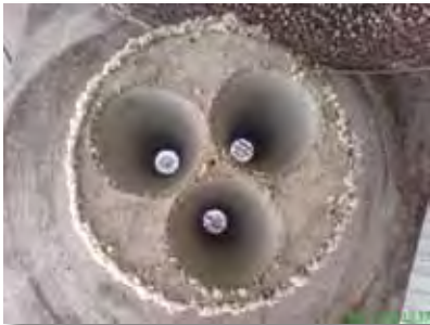
Inside the unit is clean and fully operational.
